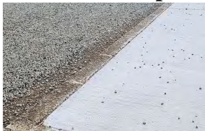
Loose chip seal - the new normal across suburban Auckland
